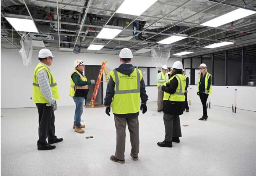
Carroll County Career and Technology Center Construction Image Source: Brian Krista, Carroll County Times
