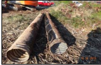
Photograph of a deteriorated metal pipe.
