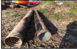
Photograph of a deteriorated metal pipe.
