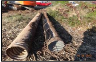
Photograph of a deteriorated metal pipe.
