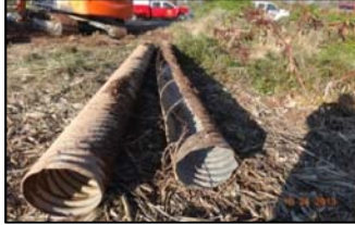
Photograph of a deteriorated metal pipe.
