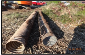
Photograph of a deteriorated metal pipe.
