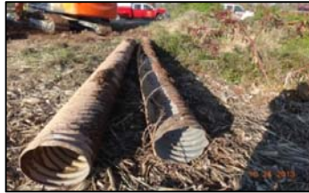
Photograph of deteriorated metal pipe
