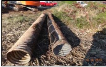
Photograph of deteriorated metal pipe
