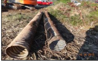
Photograph of deteriorated metal pipe
