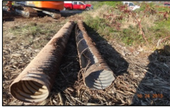
Photograph of deteriorated metal pipe
