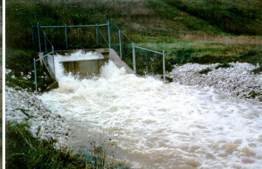
Principal spillway outlet during Hurricane Eloise (1975)
